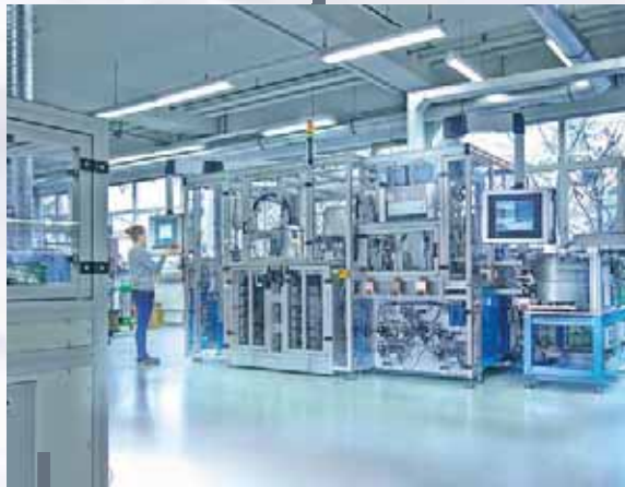
Assembly and test of pressure switches on semi and fully automated installations.
