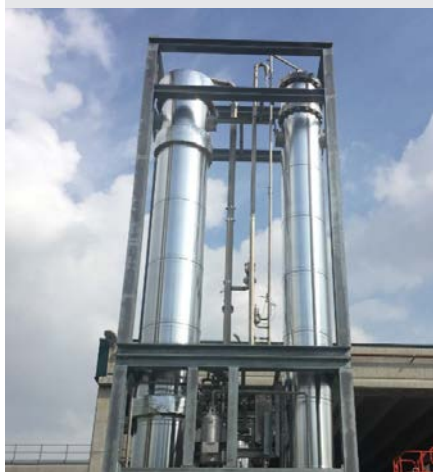
GM-GreenMethane Upgrading Unit with 125 S m3/h biomethane
