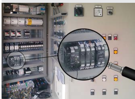
Control and command panel for underpasses with SENECA hardware and electromechanical redundancies
